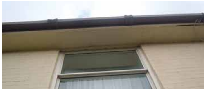
Asbestos soffit on head of window
