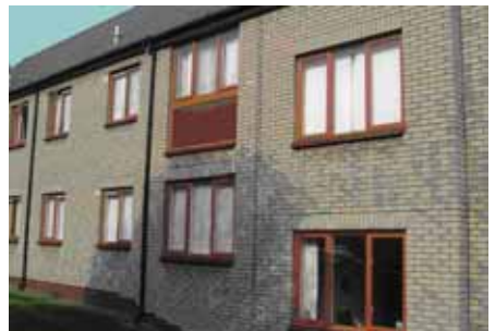
Asbestos panel in lower fixed glazing
