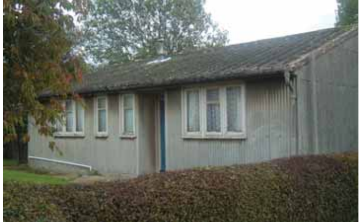
House constructed with asbestos cement sheeting to both walls and roof, guttering and down pipes are also asbestos cement
