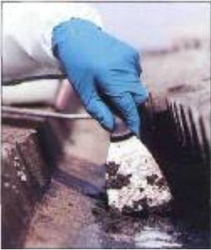
Wet the debris again if you find dry material, avoid creating a slurry
