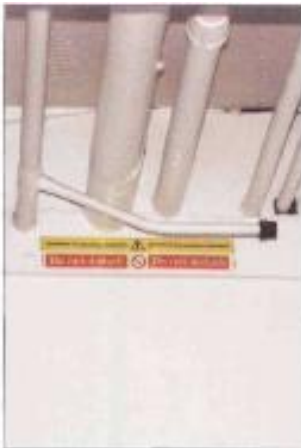
Don't assume there will always be warning signs. There could be undiscovered asbestos in buildings you work on
