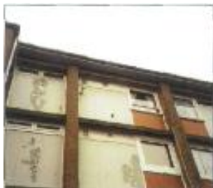
External AC panels
