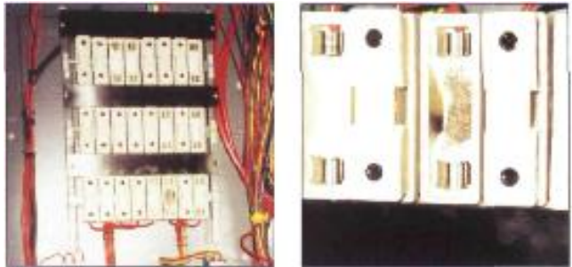
Old style fuse-boxes contain asbestos inside the fuse assemblies and must be handled correctly
