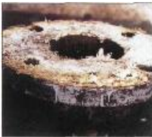
Gasket material left on a pipe flange
