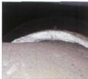
Joint packing on a flue
