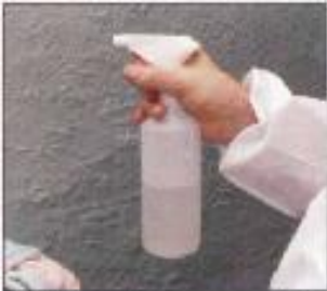
Spray at low pressure; high pressure spray could disturb fibres from asbestos paper under these tiles
