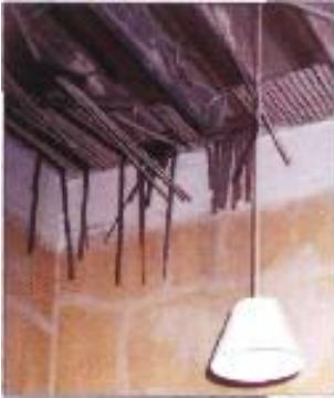
Old lath and plaster ceilings are often covered in textured coating to hide imperfections
