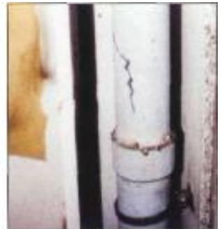
Sometimes, the joints are sealed with asbestos string
