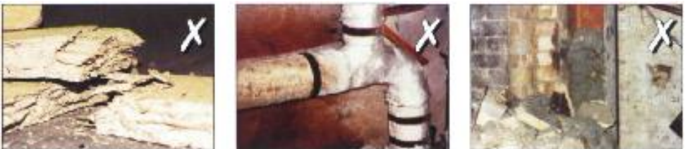
Broken asbestos insulating board, asbestos lagging and sprayed asbestos (limpet)
