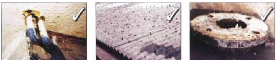
Damaged textured coating, asbestos cement roofing and an asbestos-containing gasket
