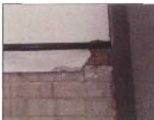
This damaged AIB needs to be covered and protected from further damage
