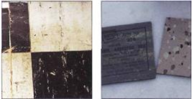
Floor tiles that contain asbestos can also have asbestos-paper backing, or be fixed with asbestos-containing mastic
