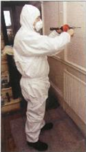
Make sure you use the right PPE for the task
